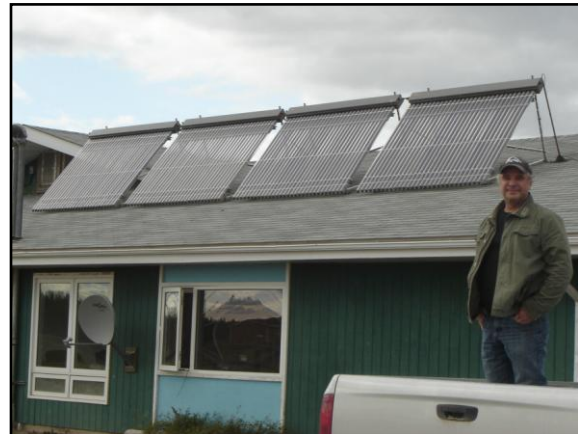
Figure 1 – SWH Tubes at Fort Providence
